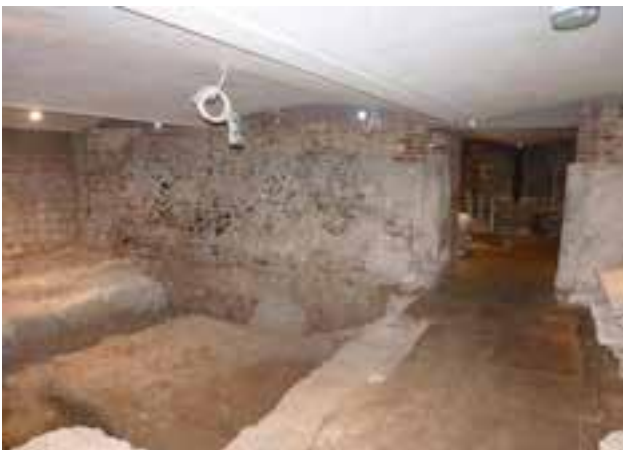
Fig 9 Archaeological investigation in front of the Norman spine wall. The 12th-century jamb is also visible.
