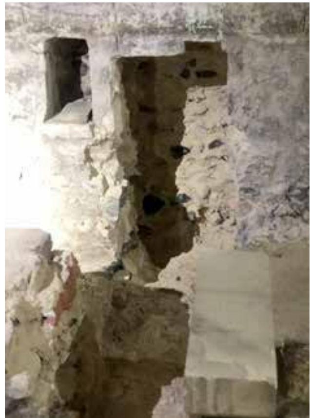
Fig 17 Formation of new pocket within wall of keep to take the new steel floor
